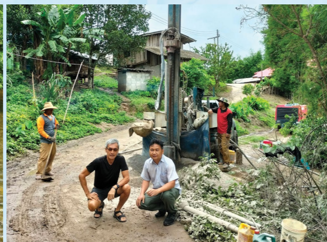
Victor working with the locals in the drilling of a water well for the village
